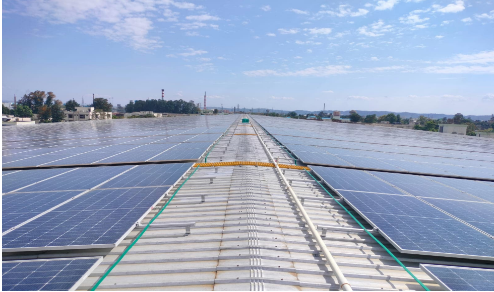
Picture: Solar Panels
